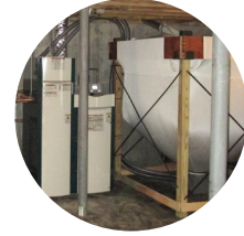
Central wood pellet furnaces and boilers
